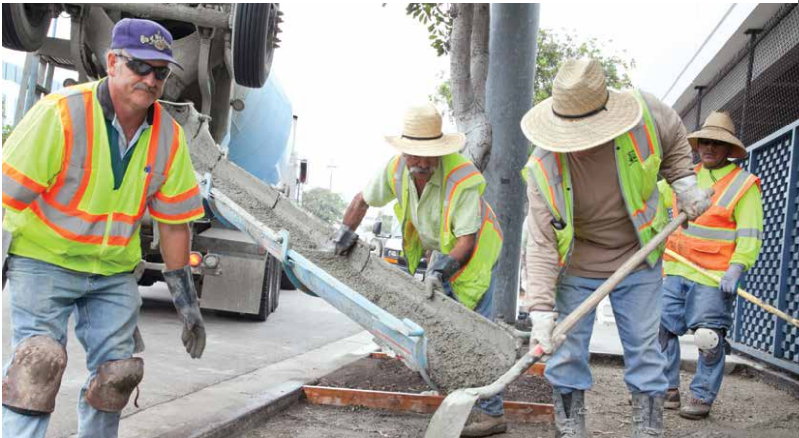
PHOTO ABOVE: Los Angeles Department of General Services replacing damaged sidewalks around the LACC in June 2014
